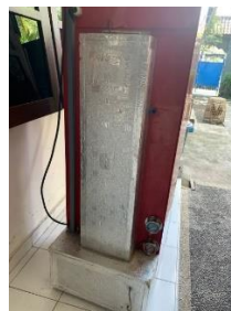
Gambar 9. Ducting tampak belakang
