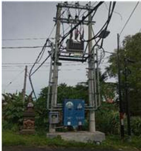
Gambar 4. 1. Transformator Distribusi BB 0092
