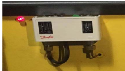
Figure 3. High Low Pressure Switch and Indicator
