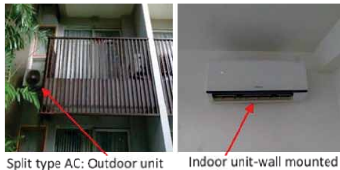
Fig. 3. Split AC system installed in residence buildings
