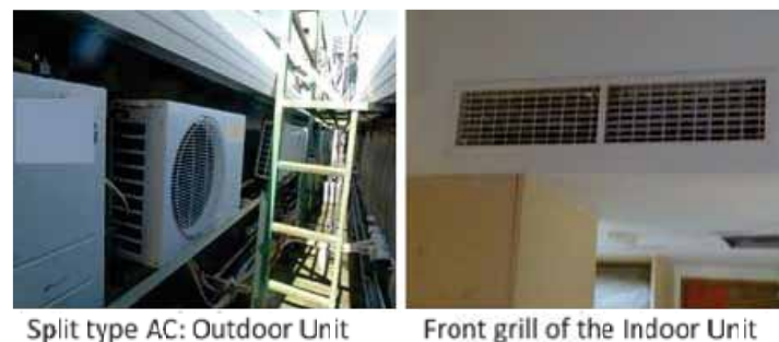
Fig. 2. Split AC system applied for Building-1
