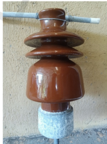
Figure 8: Pedestal insulator on clean and dry.
