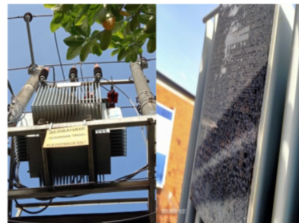
Gambar 2. (a) Gardu DB0292 (b) Name plate transformator DB0292.
