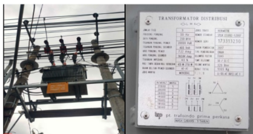
Gambar 1. (a) Gardu DB0575 (b) name plate transformator DB0575
