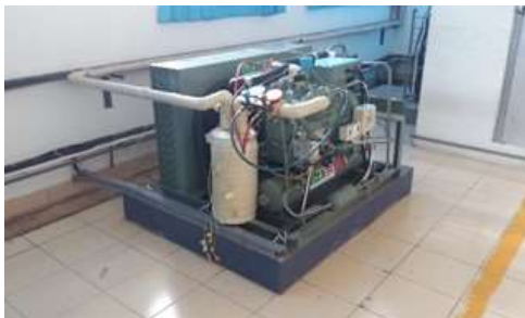
Condensing unit system cascade
