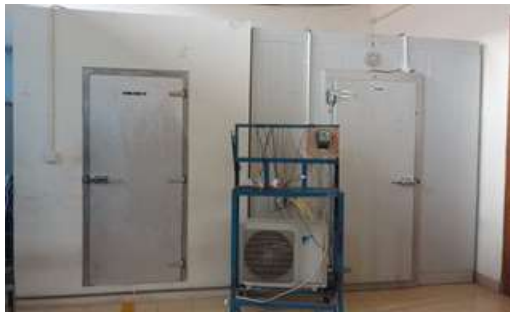
Conventional cold room system
