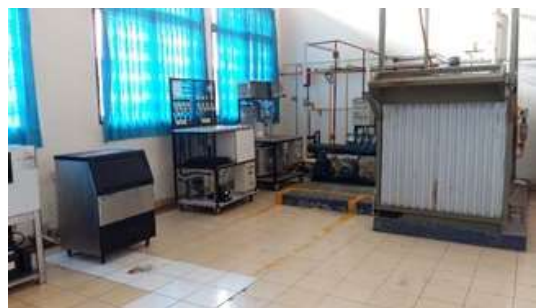
Ice machine - refrigeration system
