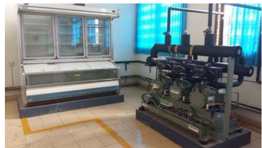
Multirack refrigeration system
