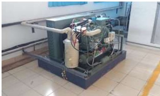
Condensing unit cascade system
