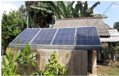
Figure 4: Solar panel used to energy source.
