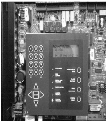
Gambar 8. MCFA (Main Control Fire Alarm)
