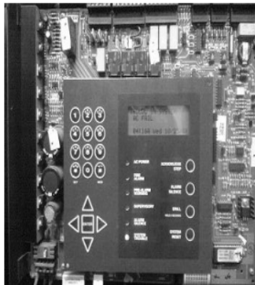
Gambar 8. MCFA (Main Control Fire Alarm)
