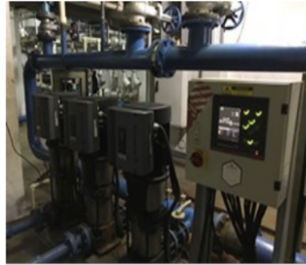
Gambar 6. Kontrol panel sistem suplai air bersih di Double-Six Luxury Hotel Seminyak
