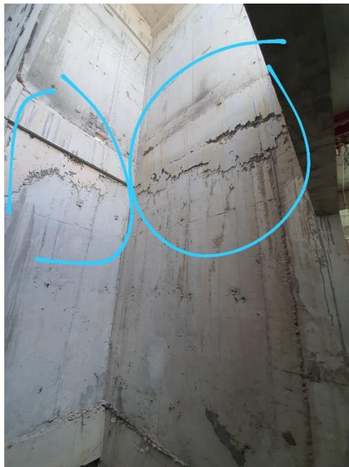
Bleberan beton pada dinding lift As 4/K-L.
