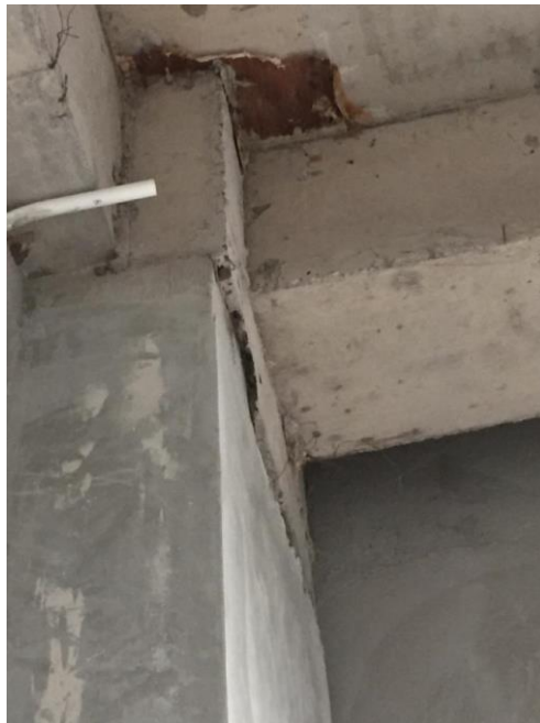
Sisa kayu bekas bekisting plat as 2/K
